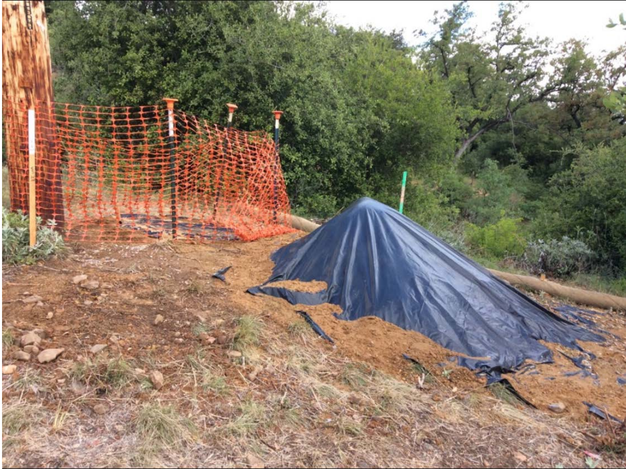
Photo 4: The pole hole and spoils stockpile at P259357 (TL 626 Conversion North (C 222)) were observed to be securely covered in accordance with MM BIO-23, and the ECP/SWPPP (MM HYD-1 and MM BIO-7).
