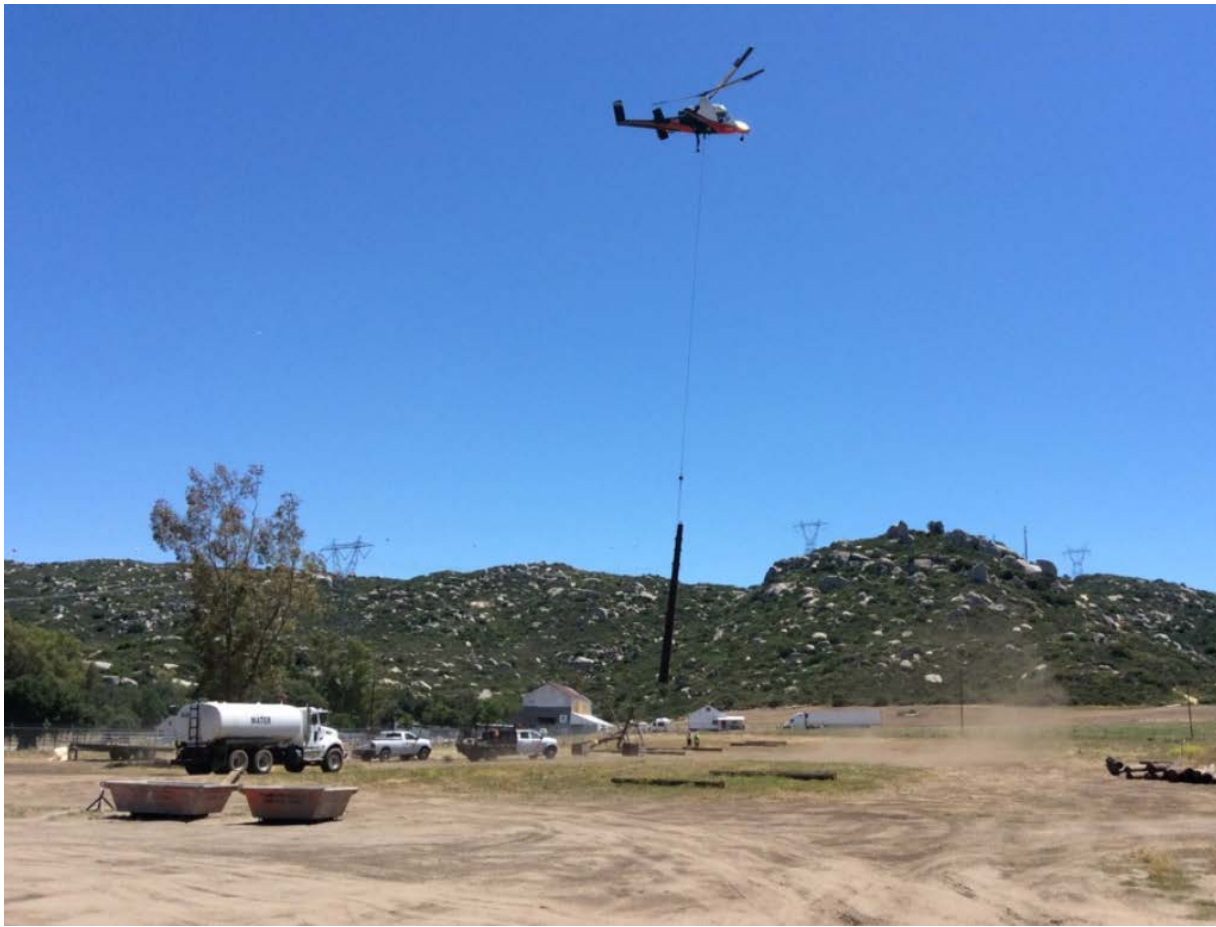
Photo 1: A crew was observed using helicopter external load operations to pick both sections of Z972820 from Sol Valley Staging Yard South (TL 6923). A water tender was observed applying water to the surface surrounding the pole immediately prior to and in between pick up to minimize dust emissions from helicopter rotor wash in accordance with APM AIR-02 and APM AIR-05.
