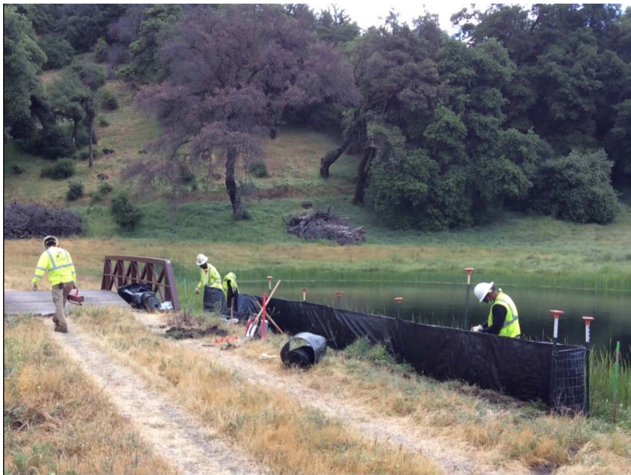
Photo 5: A crew was observed installing silt fence at P259353 (TL 626 Conversion North (C 222)) in accordance with the ECP and SWPPP (MM HYD-1 and MM BIO-7). A full set of fire tools was observed on site in accordance with the CFPPP (MM FF-1).
